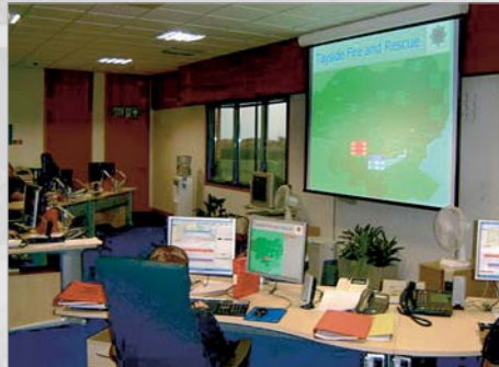
Newly-installed communications equipment in our command and control centre has enhanced our call handling and radio communications capabilities.
