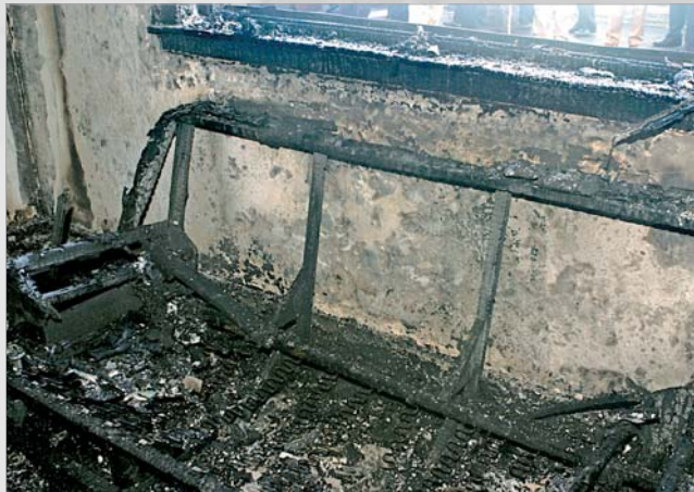
A burnt-out settee inside a flat WITHOUT domestic sprinkler protection after combustion.
