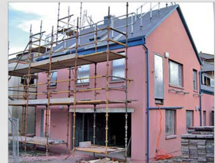
Part of Tayside Fire and Rescue's new training facility, nearing completion at Arbroath.
